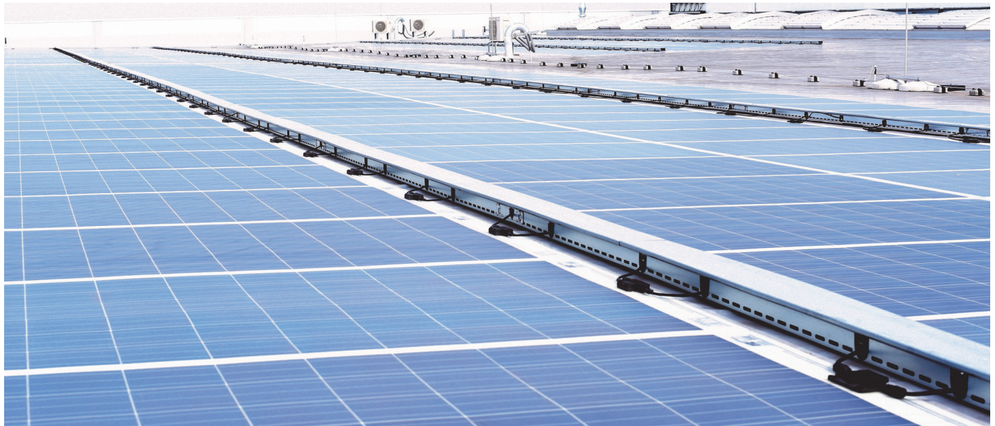
Rooftop installation DAS Energy Headquarters
